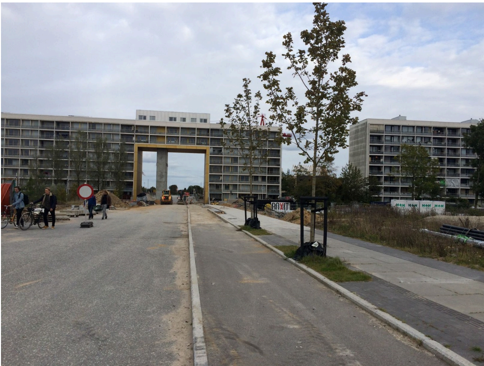
Figure 4.5. Part of the residential building block in the centre of the picture has been demolished to open up a new entrance to the Gellerup neighbourhood. The building has been kept because its prominent views give it great value. Photo: Sandra Oliveira e Costa
